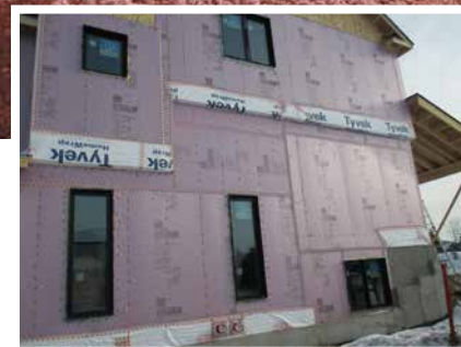
Image shown is of the Net Zero Discovery Home (Lot 7) to demonstrate the exterior air barrier system
